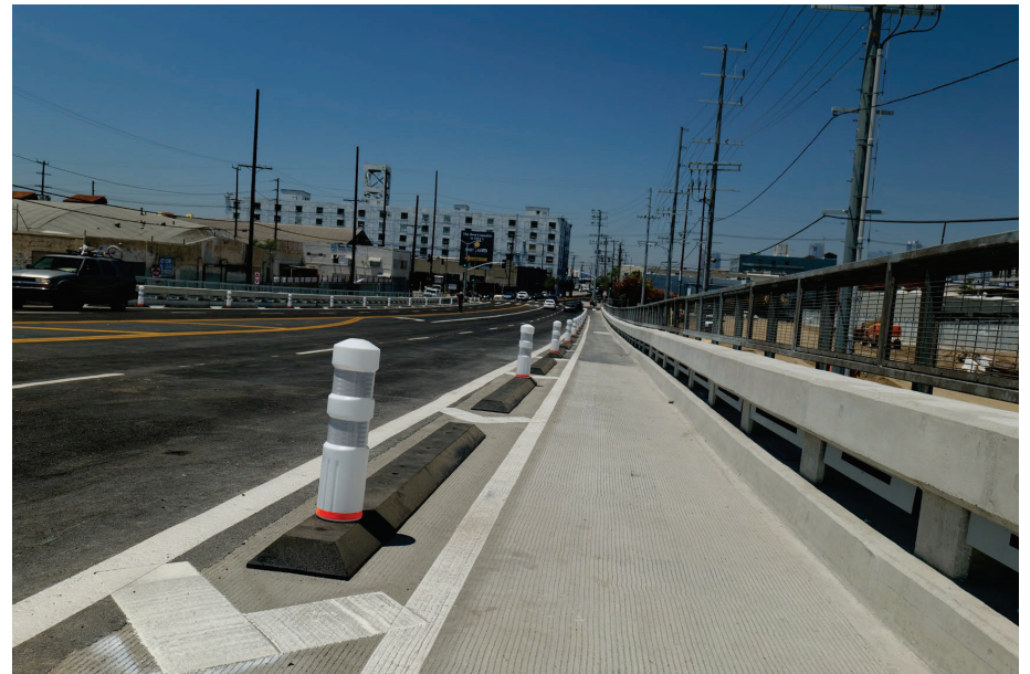
K71 Post on 4"x15" Curb
