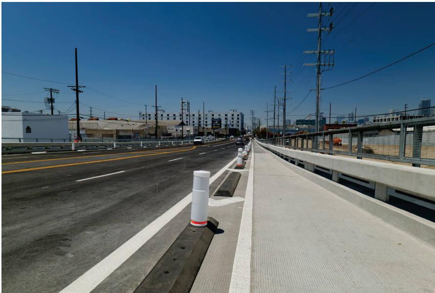
K825 Post on 4"x15" Curb
